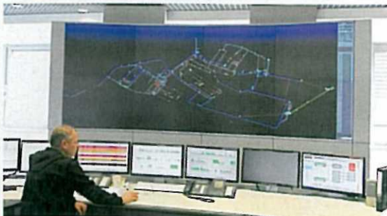
A ventilation control room combines data input with a visual display.
